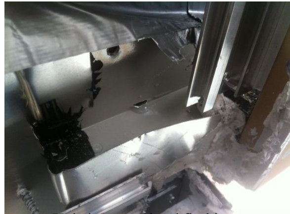
Hole in rear of head flashing
